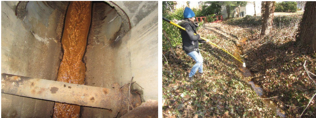
Extended monitoring in Glenwood Landing included lifting manhole covers and taking water samples from pipes running under Glenwood Road as well as from the stream that runs north of Glenwood Road (photos by Michelle Lapinel McAllister and Carol DiPaolo, 1/19/22-3/22/22)
