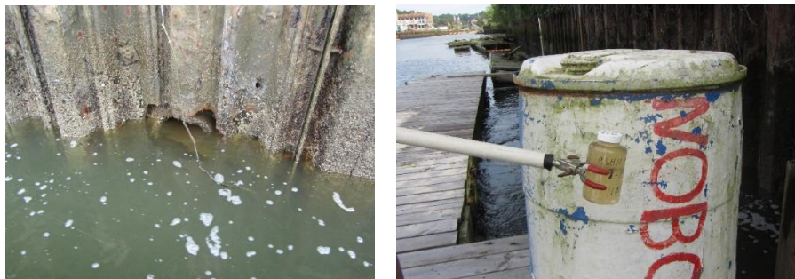
Glen Cove Creek discharges: malfunction of pump station during cleanout of the STP UV system (top, l, 7/11/18); brown discharge from north bulkhead (top, center, 7/17/18); white discharge from CSHH #10 (top, r, 10/31/18); brown discharge at CSHH #9 and water sample (bottom, 9/19/18) (photos by Carol DiPaolo)
